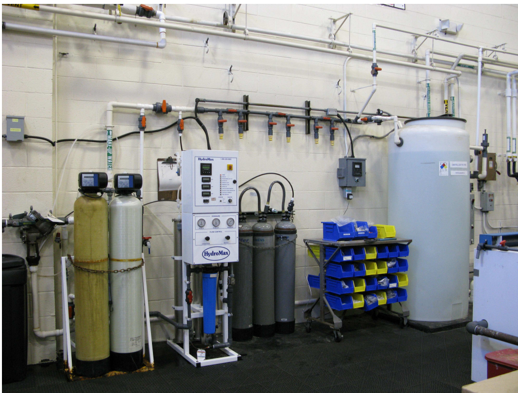
Figure 1. Electroplating Shop Reverse Osmosis/De-Ionization water treatment system.
