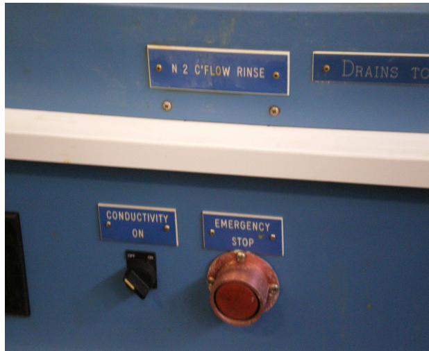
Figure 7: Cold water rinse tank conductivity probe switch "Off."
